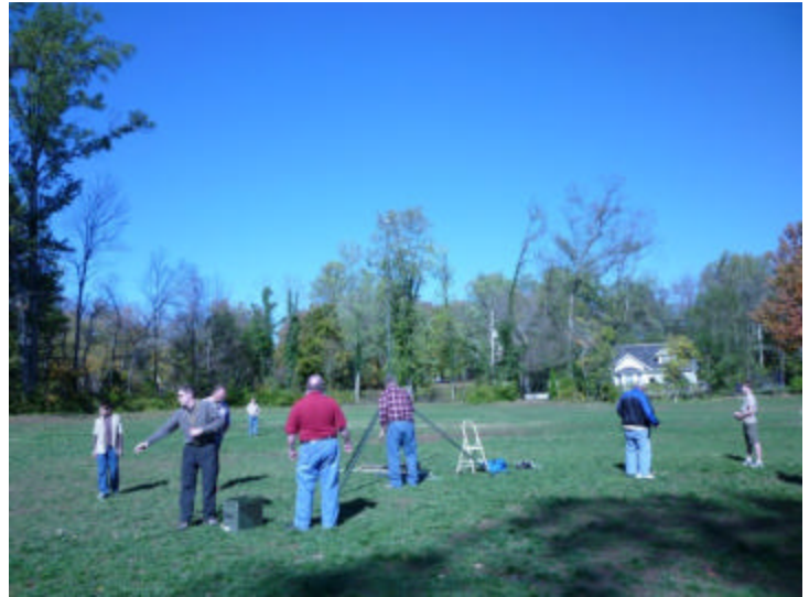
The beginnings of the main mast for the HF antenna begin to take shape with scouts at the ready.
