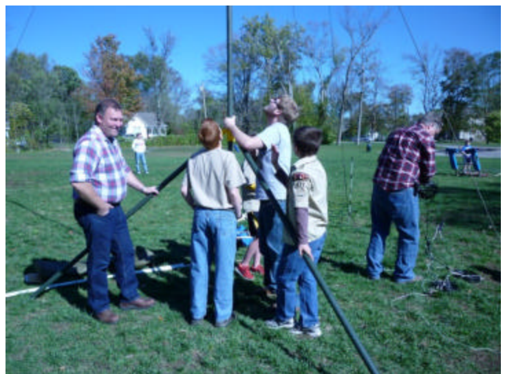
All hands are needed to steady the mast base (above). 2nd mast is erected for HF feed-line & dual-band antenna (left).
